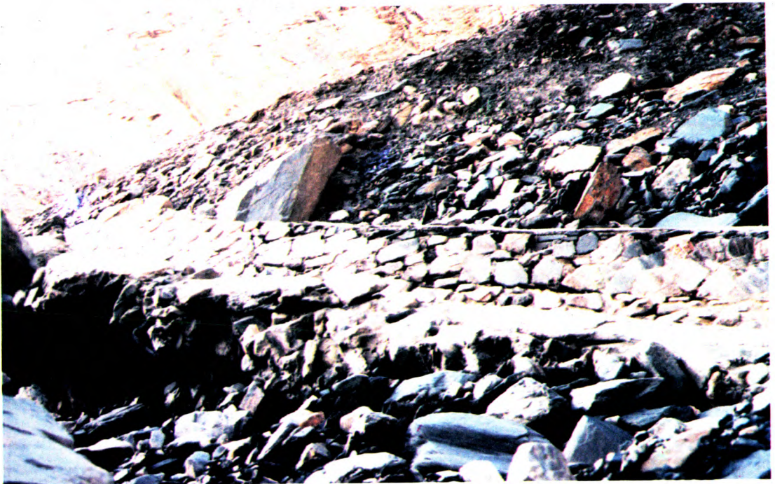
PLATE - 24 Another view of the damaged water drain due to change of nullah course of mudflows slide No. 12.
