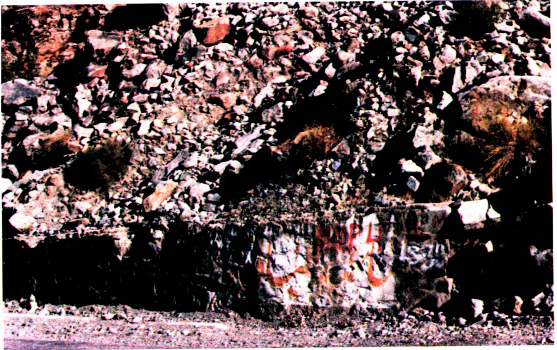
PLATE - 23 Mudflow slide No. 12 showing the damaged water drain to change of nullah course because of mudflow.
