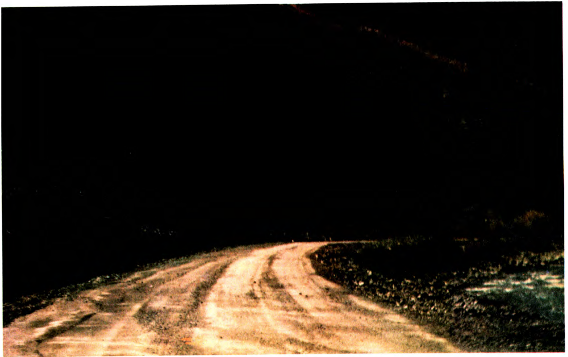
PLATE - 25 Damaged toe wall at the river bed level at the site of GSP slide No. 13.
