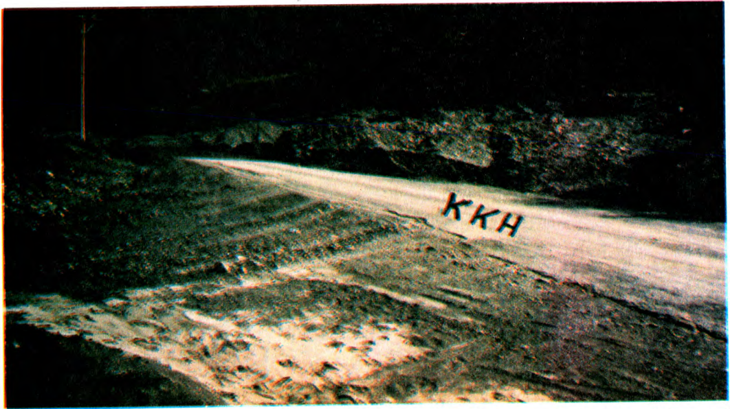
PLATE - 13 GSP slide No. 7 showing the scree material piled up on both sides of the road.
